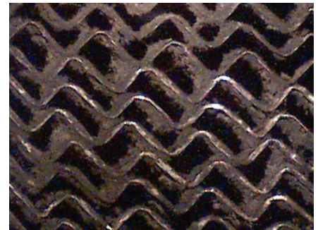
FIGURE 3: Ten times magnification of core 1, the untreated sample after the simulated 4 years of heavy ETS loading. The buildup of ETS is clearly visible, with perhaps 20% of the flow area blocked.
